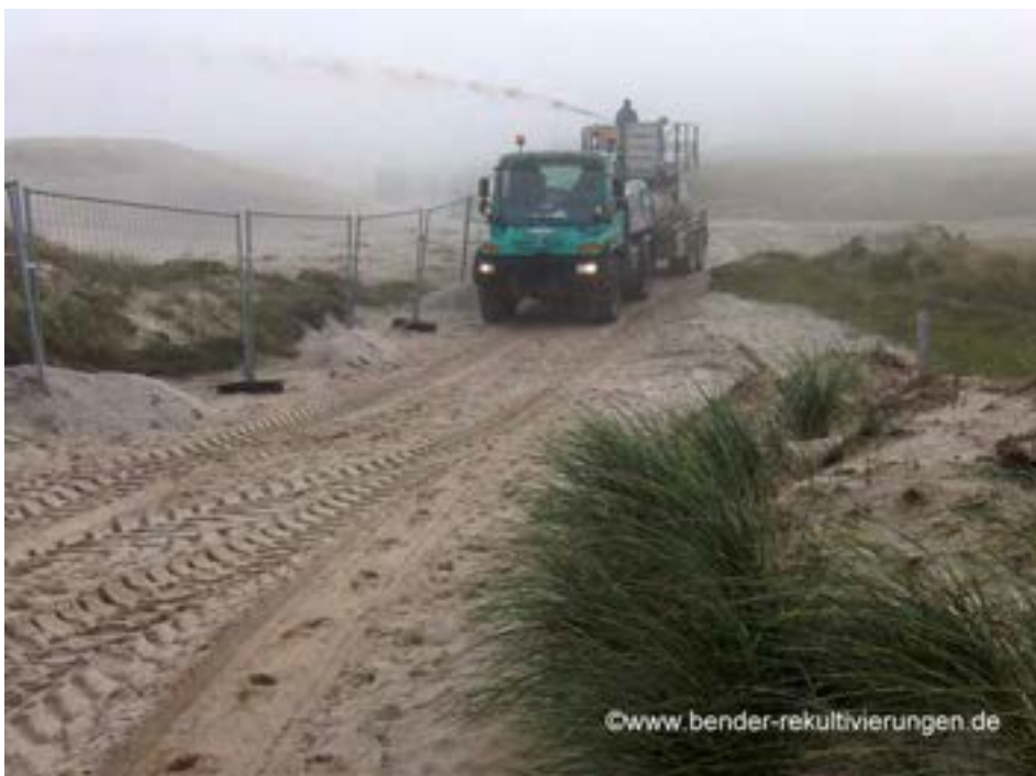
Figure 60. Surface stabilization for dust control at an industrial site using soil binding agents applied by a hydroseeder
