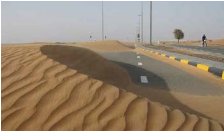
Figure 50. Damage to infrastructure by moving sand dunes
